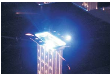
Welding of the tube / base plate joint of an exhaust gas heat exchanger utilizing a beam scanning optics
